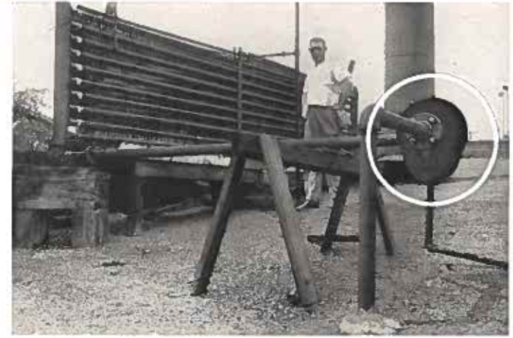
Type "S" Horizontal Oil Separator on the Roof of an Indiana Laundry
