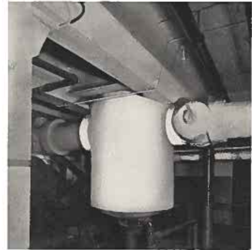
14' Horizontal Separator Handling 20,000 Lbs. of Steam per Hour at 250 Lb. Pressure 150° F. Superheat, Installed Close to Ceiling
