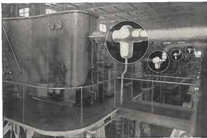
Six Type "E" Horizontal Live Steam Separators in Cleveland City Water Works, Cleveland, Ohio
