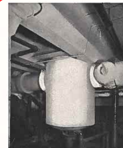
14" Horizontal Separator Installed Close to Ceiling. Handles 20,000 Lbs. of Steam per Hour at 250 psi and 150° F. Superheat.
