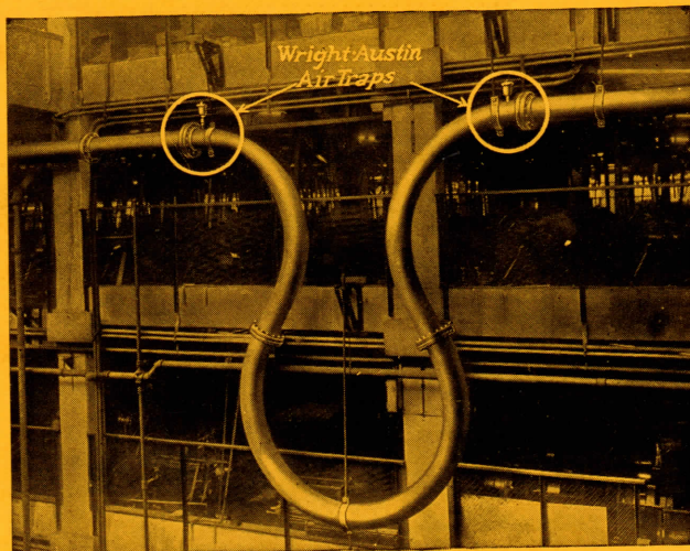
Several Hundred Air Traps are used on Hot Water Heating System in Plant of Ford Motor Company, Detroit
